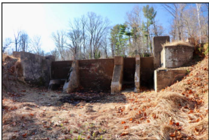
Photo 1 The dam had several leaks before work began.
